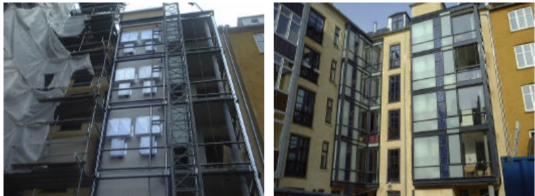
Figure 4.3.: The ventilation system is installed outside the external wall.
