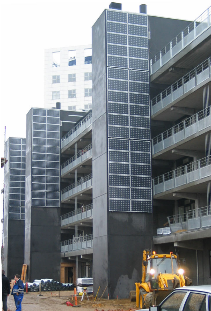
Figure 3: 200 m 2 PV modules have been mounted on the towers in the housing project Dalgasparken in Herning with 72 apartments.
