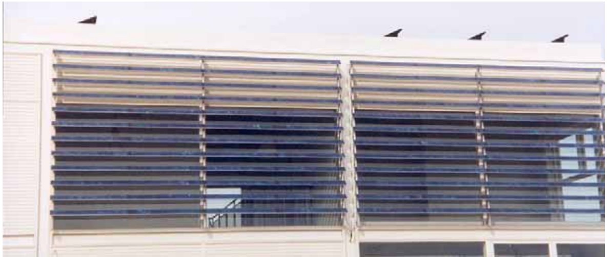
PV shading systems (ALU-PV) at students house in Herning
