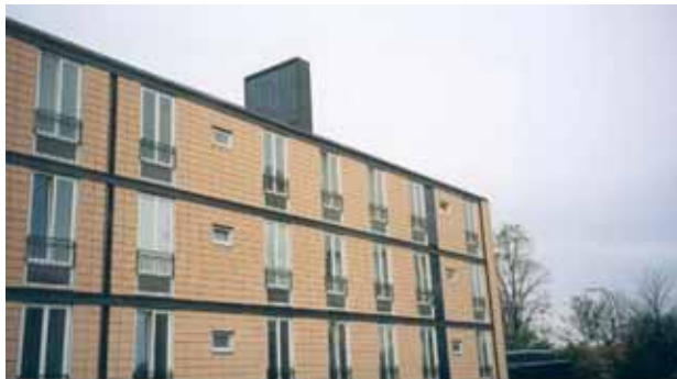
PV on ventilation chimneys at Lundebjerg Skovlunde
