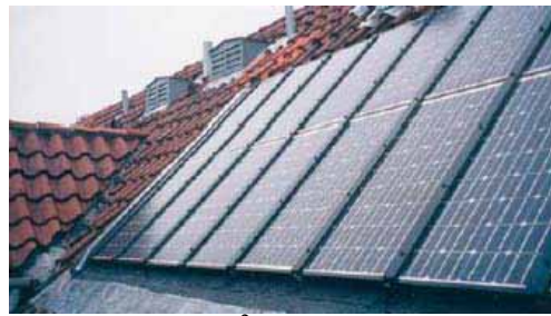
Figure 17. 200 m 2 PV panels integrated in the south facing roof.
