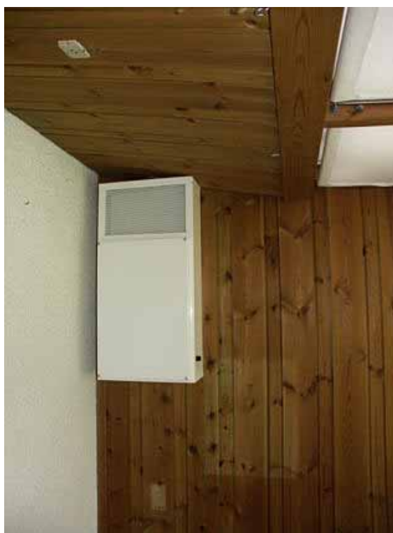
Figure 12. PV assisted ventilation system.
