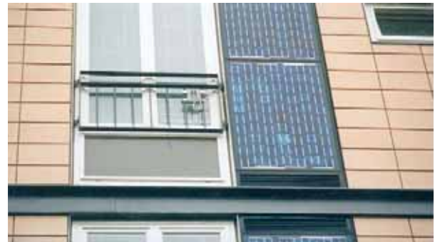
PV panels in facade
