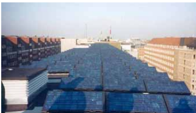
PV panels on flat roof at union SID head quarters in Copenhagen
