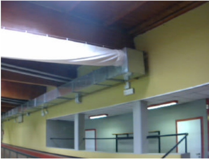
Pioltello: internal air distribution system
