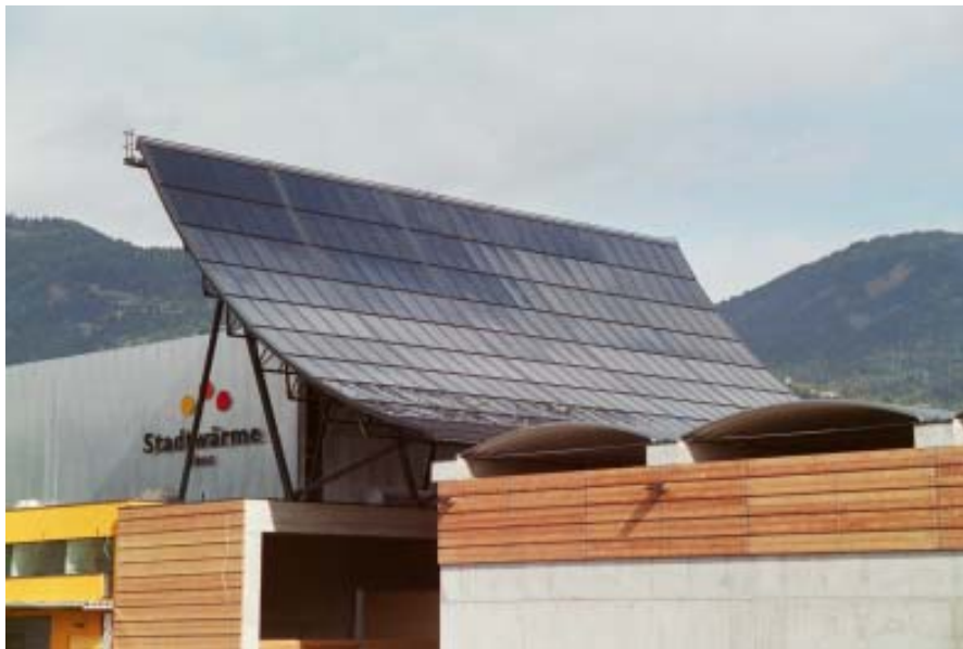
Figure 1: The solar supported biomass heating network in Lienz, East Tyrol, (630 m 2 gross collector area) was taken in operation in 2002 (source: S.O.L.I.D.).
